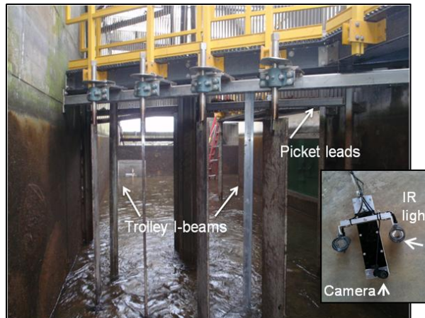
Figure 1. Left: McNary North fish ladder picketed lead section, looking downstream. Picketed leads are shown in the raised position typical during winter maintenance. Inset: video camera trolley system with stabilization weight (black), armored cable, adjustable lights and video camera.
