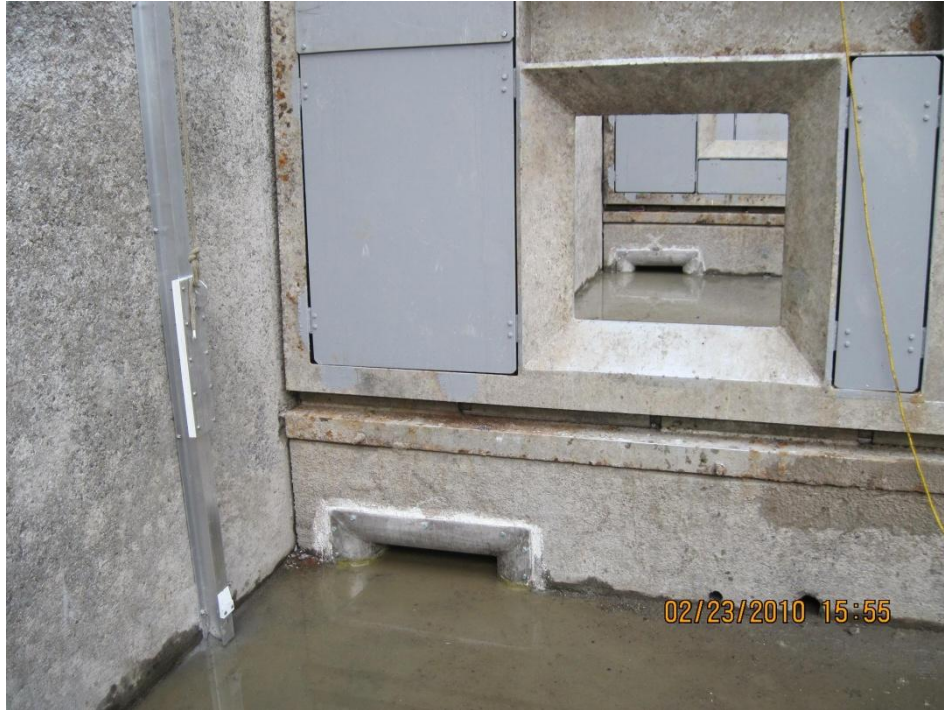
Figure 3. Dewatered McNary south ladder, facing upstream, 2010. A lamprey orifice is visible at lower left, and a fish passage orifice is visible at upper right. A camera placement I-beam is shown against the left ladder wall. Although this orifice and camera rail were not part of the 2013 study, the relationship of the camera-mount I-beam to the lamprey orifice is illustrative of other orifice locations monitored in 2013.
