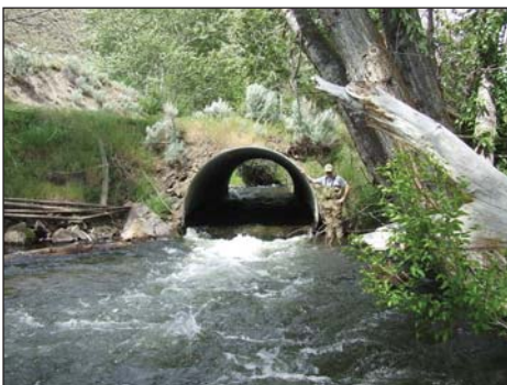
Before: Culvert on Iron Creek prevented juvenile access to upstream habitat.
