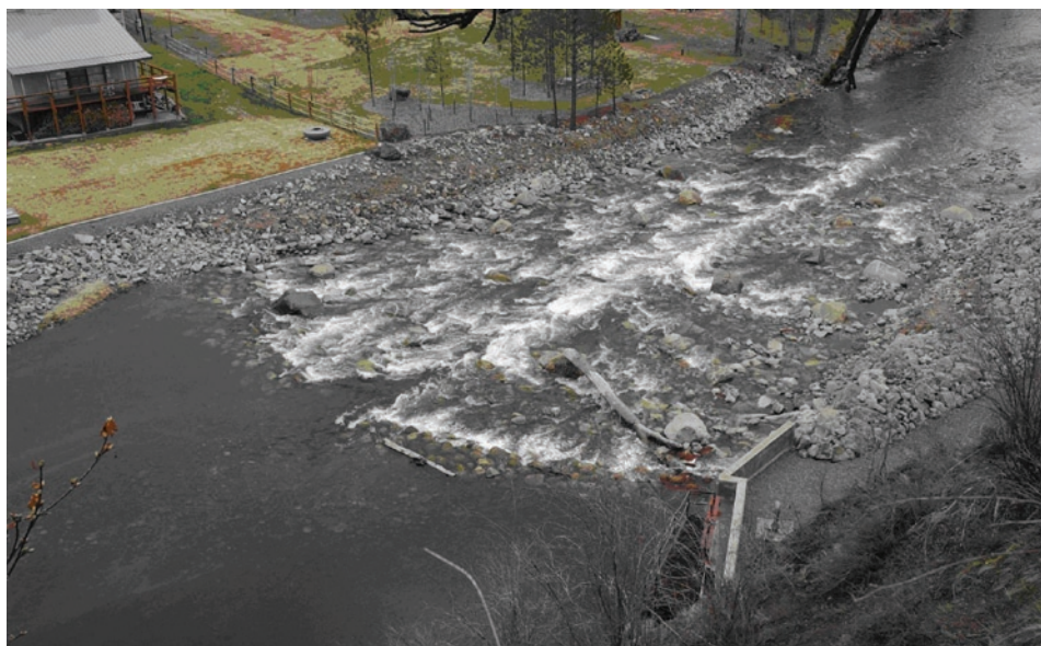
Fulton Diversion Dam (After). Low streamflow is concentrated down the center of the completed rock ramp.
