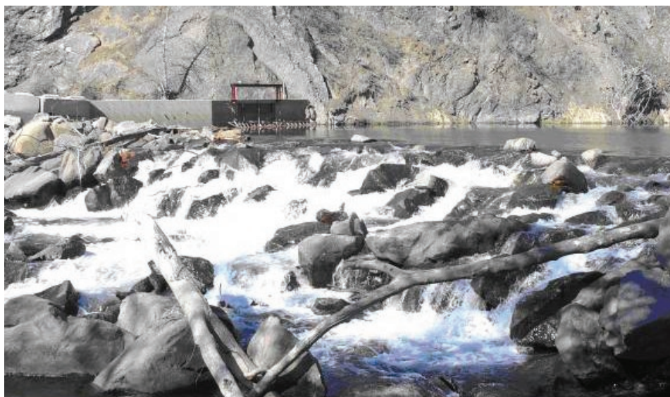
Fulton Diversion Dam (Before). The boulder push-up dam was a barrier to fish passage.
